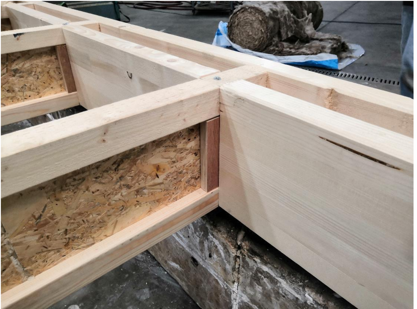
Photograph 3 – Detail of the void fillers in-between the joists and timber blocks Note: Photo taken prior to fixing with nails
