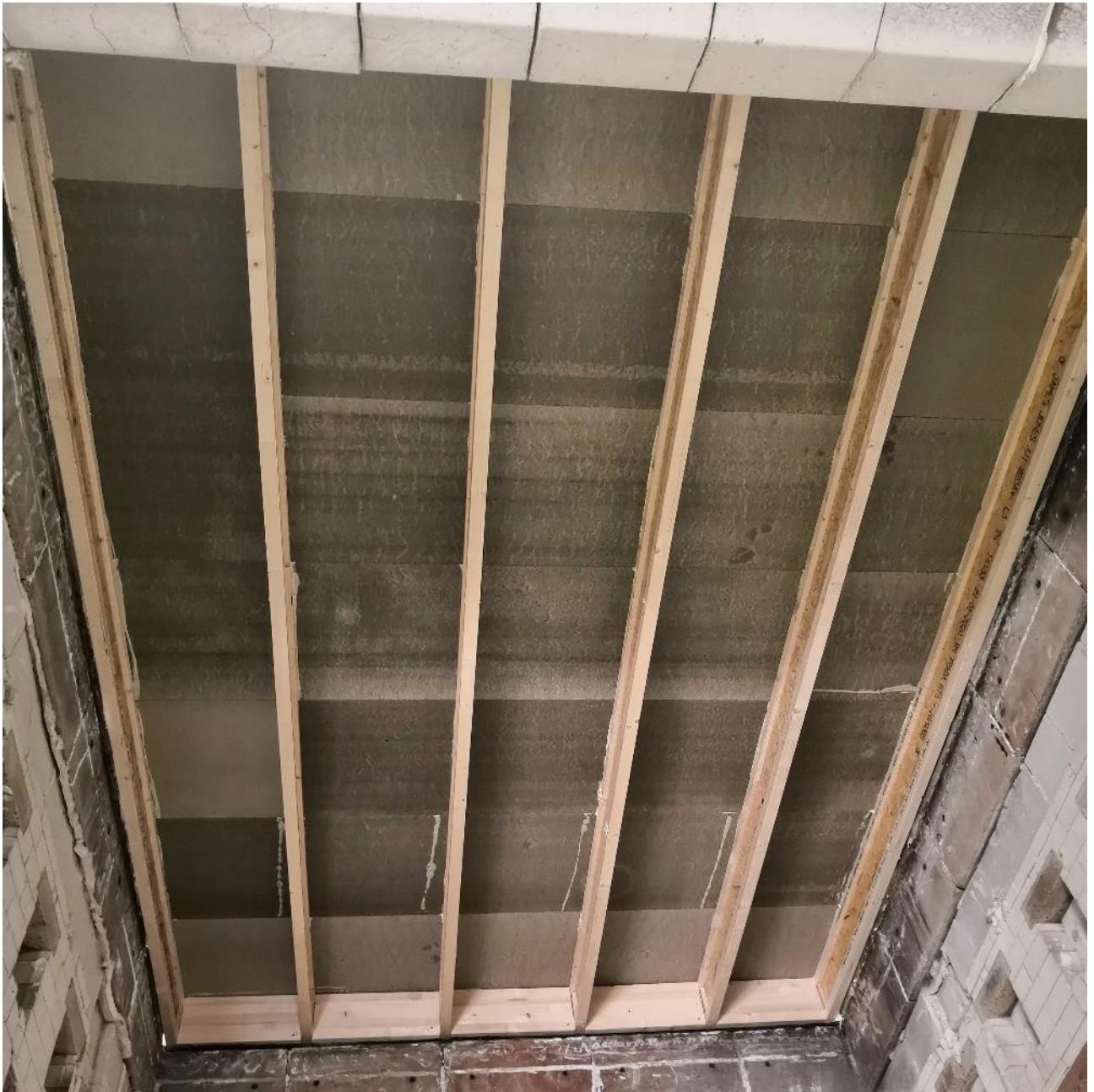
Photograph 6 - Overall view of the exposed side of the CaberFloor P5 layer before the installation of the Gyproc Plasterboard layer
