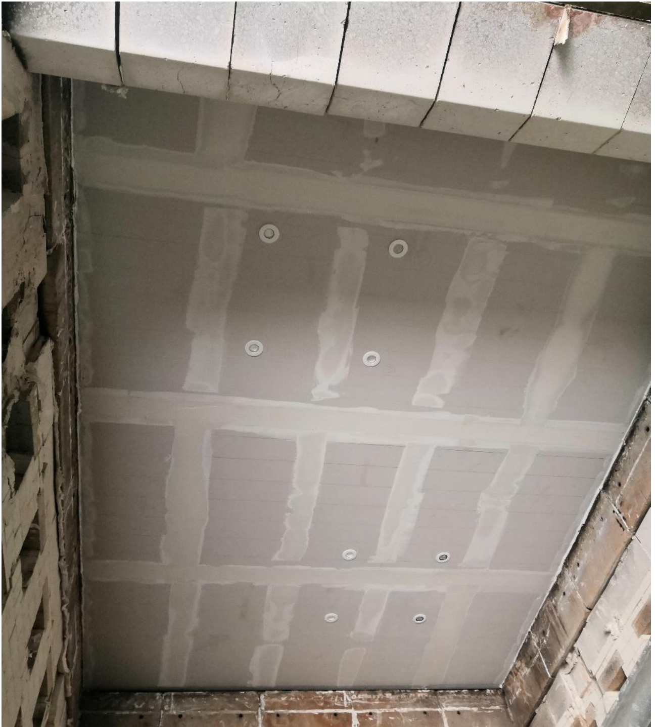
Photograph 7 - Overall view of the exposed side of the Gyproc Plasterboard layer, showing the general position of the downlighters.
